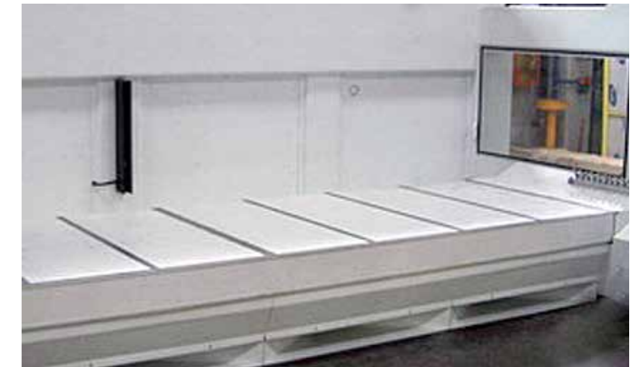
Dust extraction vents
